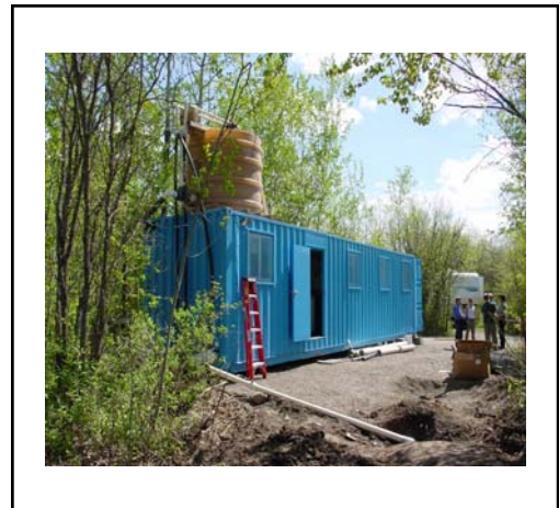
Pilot conservation hatchery under construction in late May 2006 Vanderhoof, BC. The FFSBC got the
